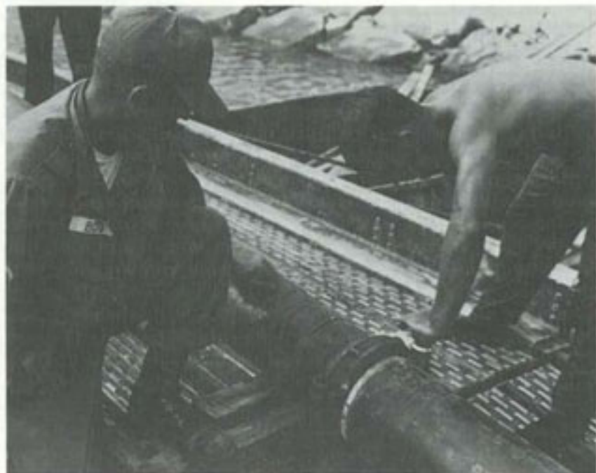
FUEL PIPELINES stretched 270 miles through Vietnam.
