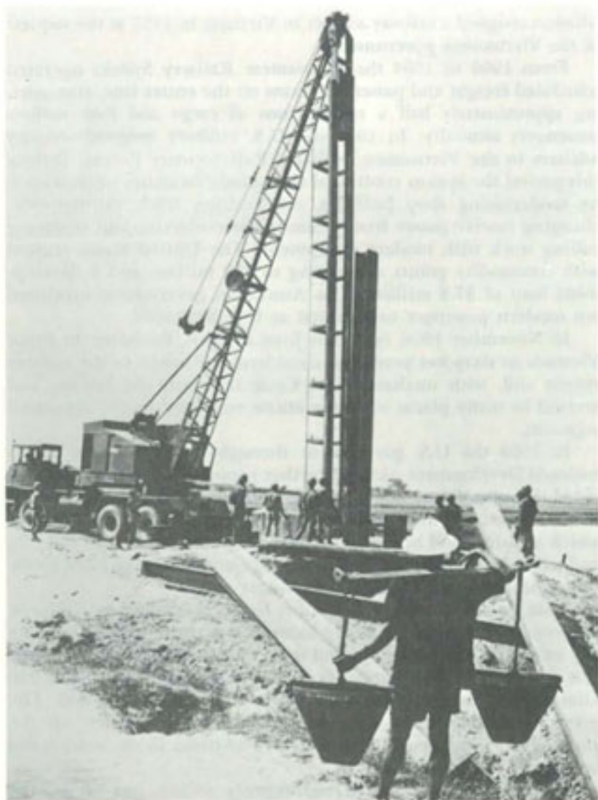
VIETNAMESE ENGINEERS drive piles for a bridge span near Qua Giang with new American equipment.
