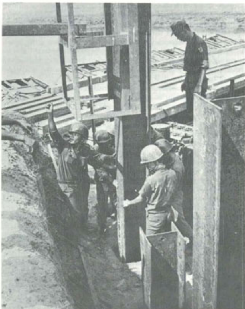
CORPORAL MUNG, 103d Engr. Bn., ARVN, directs his construction crew in pile driving for a new bridge.
