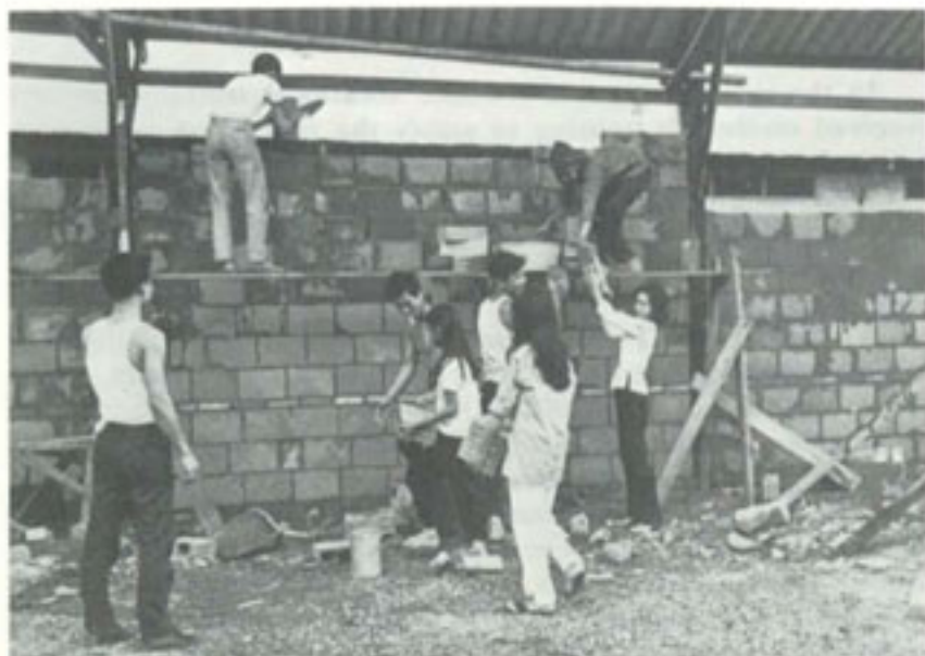
STUDENT VOLUNTEERS help construct a dormitory for war orphans at the Buddhist Institute, Saigon.
